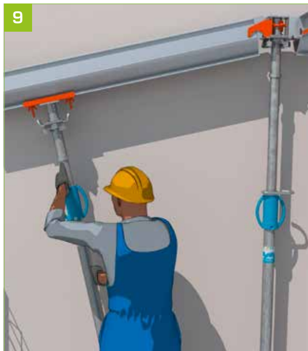
- Lift the primary beam using the technical support inserted into the FSAB.
