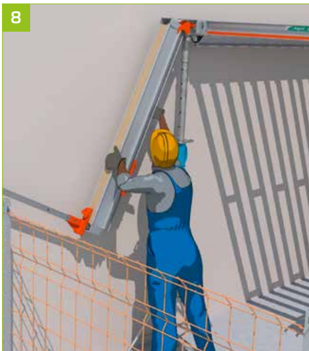
- Suspend the equipped primary beam by inserting it into the new-generation bracket.
