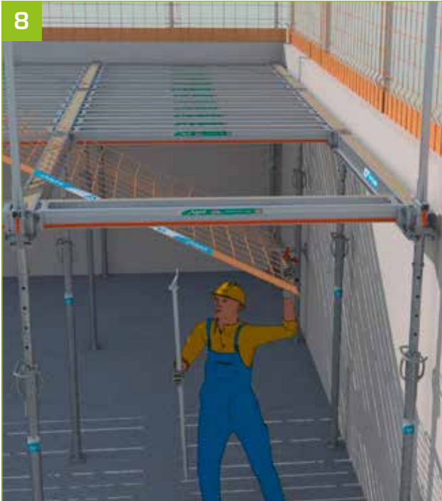
- Install the AlphaSafe mesh of less than 15 kg by sliding it over the formwork, with the baseboard on the post side and the self-adhesive label facing upwards.
