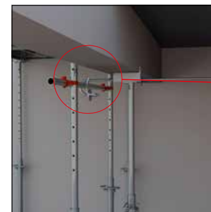
- Set up the stabilisation of the first components. - Once in place, the tripods can be removed.
