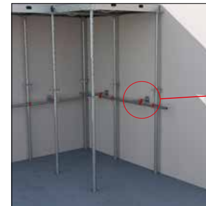
- Set up the stabilisation of the first components. - Once in place, the tripods can be removed.
